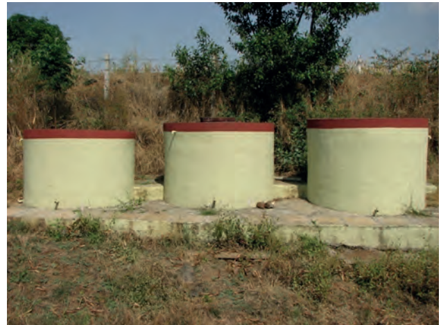
Rainwater harvesting tanks
